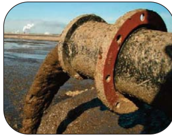
Ore & Slurry Pipeline Systems
